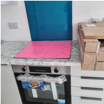
5.1.5 Hi-vis protection on an induction hob
